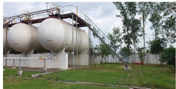
Figure 7.1: Satellite Plant of BM Energy BD in Bogura (Source: Google Map)
