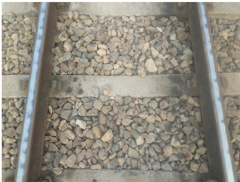
Fig. 3: Rail Track with Missing Fasteners
