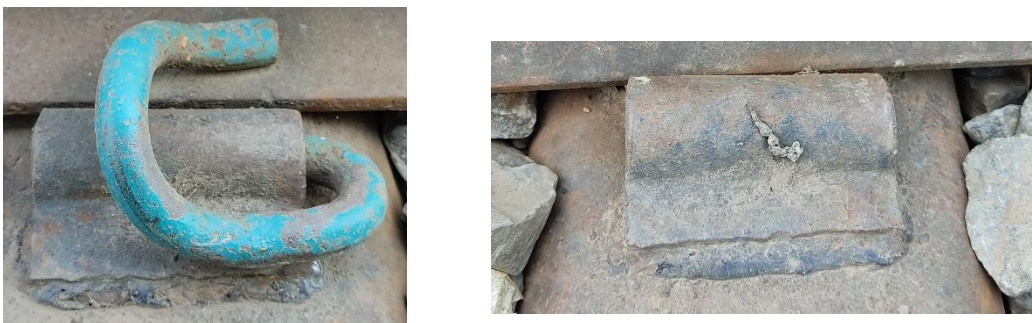
Fig.9 &10: Fasteners and Missing Fasteners
