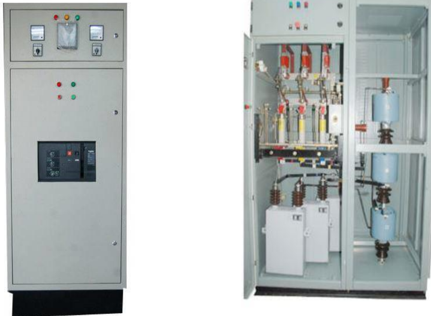
Fig 2.4: HT Switch gear
